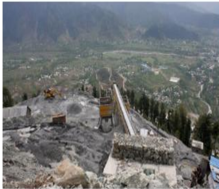
Work in progress on the Kishen Ganga Hydro Electric Power Project in North Kashmir district of Bandipora in 2012. NISSAR AHMAD
